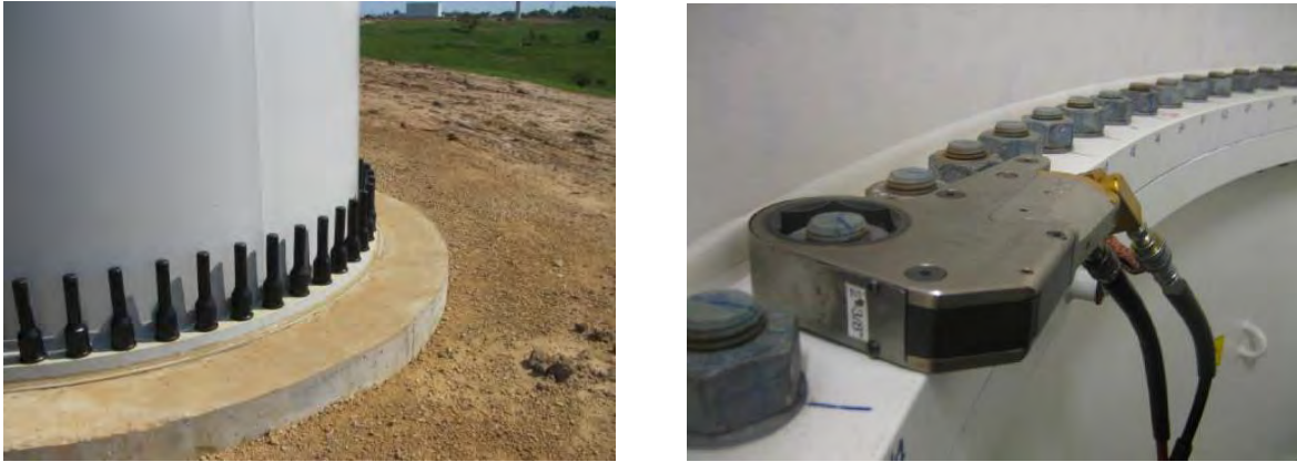
Figure 2.15: Use of Bolted Connections in Current Tower Designs (Gundersen Envision, 2013; NIB Torque, 2013)
