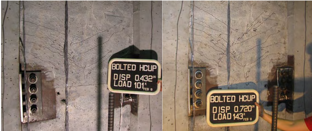
Figure 4.34: HCUP-BC Operational and Extreme Panel Cracking
